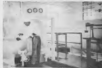
An important part of the refinery never seen by the average employee is the Ethyl Blending Plant, where (clockwise) lead, a colored liquid, is added to gasoline to raise its octane number (increasing its power). Above, Joseph Coormen is springing a "weight tank" to add the fluid to a meter gasoline blend. The big tank behind him is suspended on a delicate set of scales, so the amount of Ethyl fluid added can be accurately controlled. The gasoline blends are first tested by the Laboratory to determine the amount of lead to be used, which ranges from a maximum of one and a half cubic centimeters per gallon in motor gasoline to a maximum of three and a half cubic centimeters per gallon in aviation gasoline.
